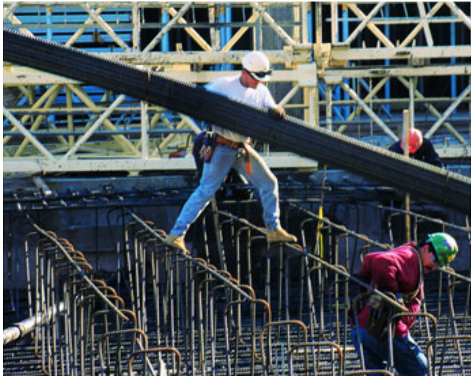
A pre-job risk-assessment strategy can alert contractors to these and other worksite dangers.
